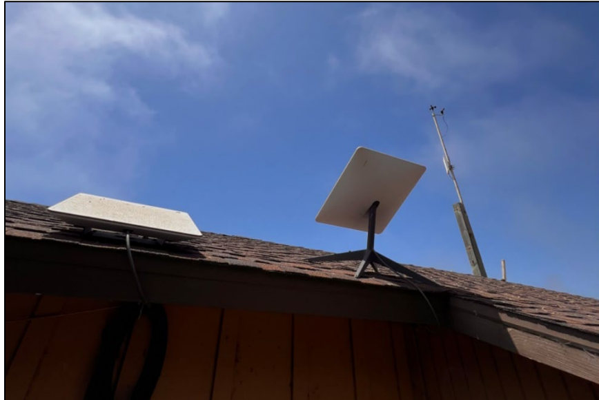
Figure 1. Starlink Dish Installed at Jalama Beach County Park
